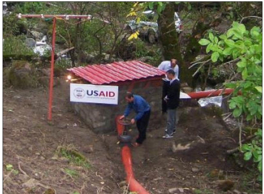
Construction at Gadamshi consisted of laying 250 meters of penstock pipe, installing 2 prototype 4.5 kilowatt turbine-generators and 1,250 meters of power lines to connect the village households.
