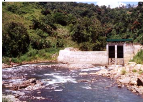
Bubunawan 7-MW mini-hydro project powers Cagayan de Oro City & vicinities in Mindanao
