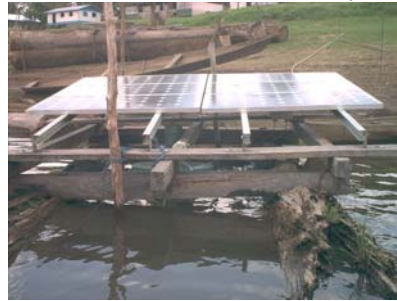
Floating PV panels in Mamirauá
